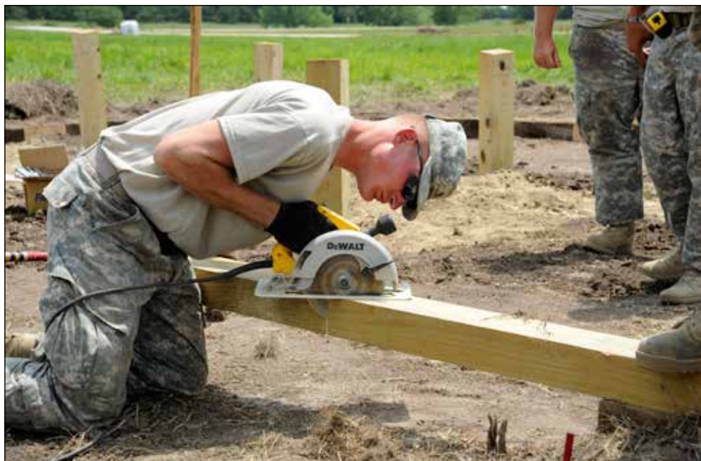
Saw Job: A Soldier assigned to the 623rd Engineer Company (Vertical Construction) uses a saw to cut a post for one of the 18 obstacles being built for a new course at Greenlief Training Site near Hastings, Neb.
