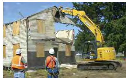
Workers remove a panel from a building at Fort Lewis, Wash., during modular deconstruction. Photo by Rebekah Barker. Date: Feb. 05, 2007. Photo courtesy of US Army from: http://www.army.mil/images/2007/02/05/2394/ .
