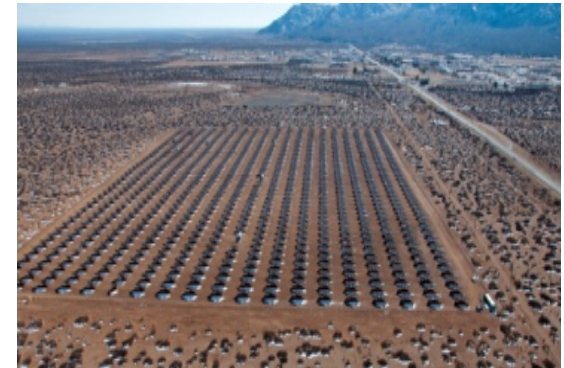
4.1 MW Solar Array White Sands Missile Range
