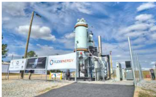
250KW Methane Power Plant Ft. Benning GA
