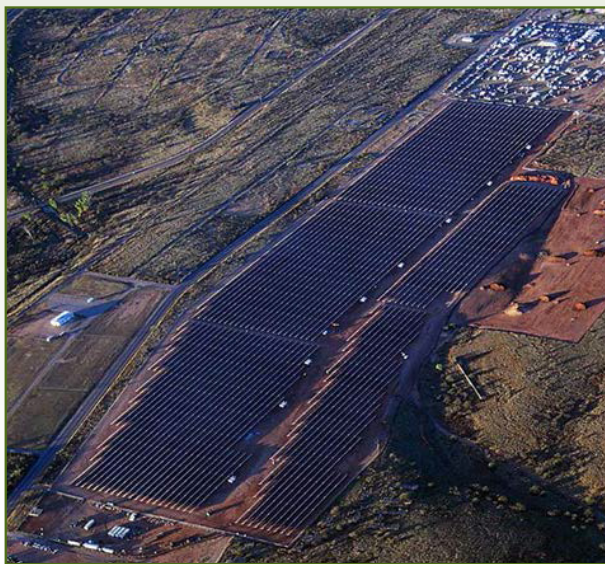
The Fort Huachuca Arizona Solar Project is operational with more than 57,000 solar panels supplying the installation and the Southern Arizona grid with renewable energy electricity
