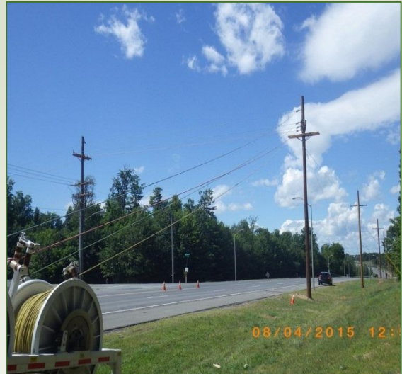
Construction of overhead lines, to be complete by spring 2016, will provide the interconnection for two substations for the BGF on Fort Drum. Photo Released by ReEnergy Holdings, LLC
