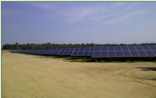
Solar panels installed at Fort Benning, Georgia
