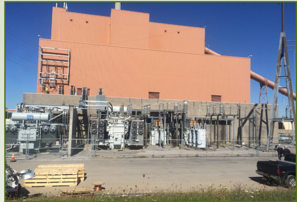
The completed substations at Fort Drum, NY. To the right stands the interconnection to the 115 kilovolt transmission grid.
