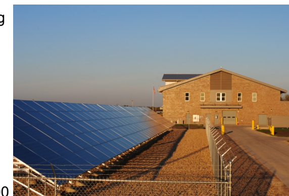
Solar panels at Joliet, IL, Army Reserve Training Center (Cpl. Scott Olijar, DVIDS)
