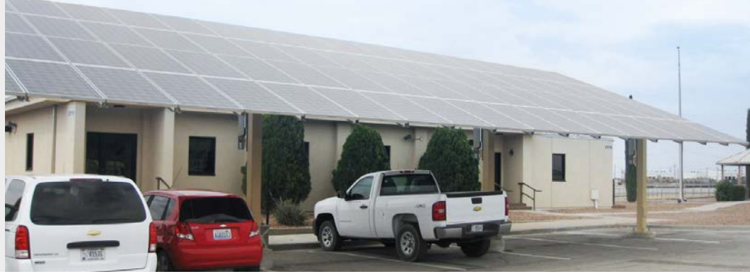
Figure 15. Carport PV Photo by Scott Huffman, NREL
