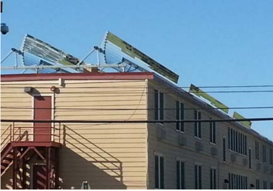
Figure 8. Cogenra ESTCP Photo by Caleb Rockenbaugh, NREL
