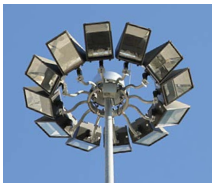
Figure 50. High mast lighting (12 kW) Photo from Sierra Army Depot
