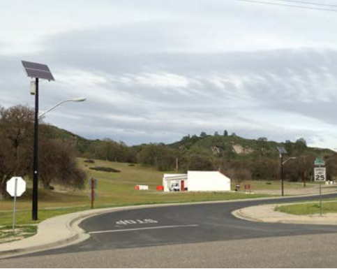
Figure 33. Phase 1 and 2 PV, solar street lights. Photo by Lars Lisell, NREL
