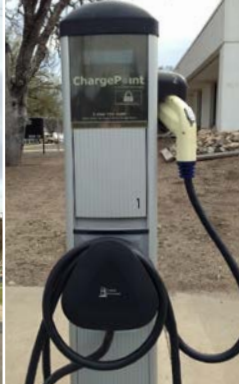
Figure 34. Electric vehicle charging station. Photo by Lars Lisell, NREL
