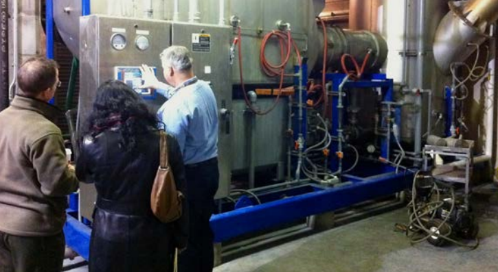
Figure 26. The NREL team inspects part of the incinerator boiler system Photo by John Nangle, NREL
