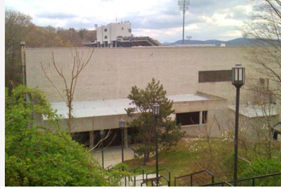
Figure 55. South wall of Hollender Center, a potential SVP building Photo by Dylan Cutler, NREL
