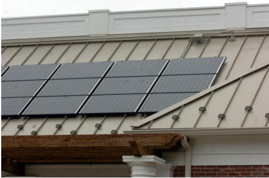
Figure 59. Rooftop solar panels on the Fairfax Village Center. 140
