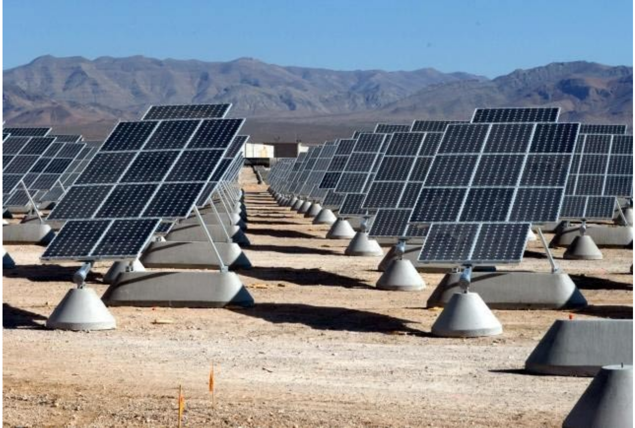
Figure 91. Solar array on Nellis Air Force Base. 141
