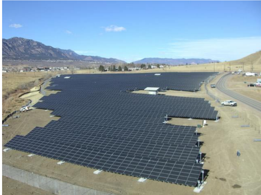
Figure 86. Fort Carson solar array. 170
