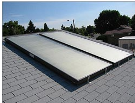
Figure 64. Photograph of a flat plate collector. 148
