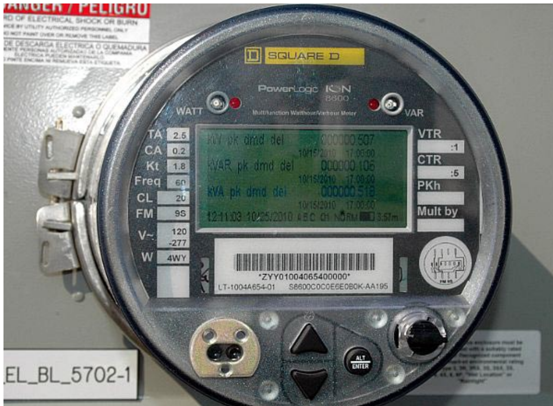
Figure 175. Advanced electricity meter installed at Naval Air Station Kingsville. 359
