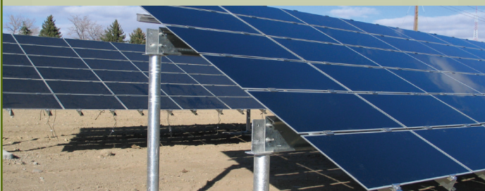
Ft. Carson Solar Array
