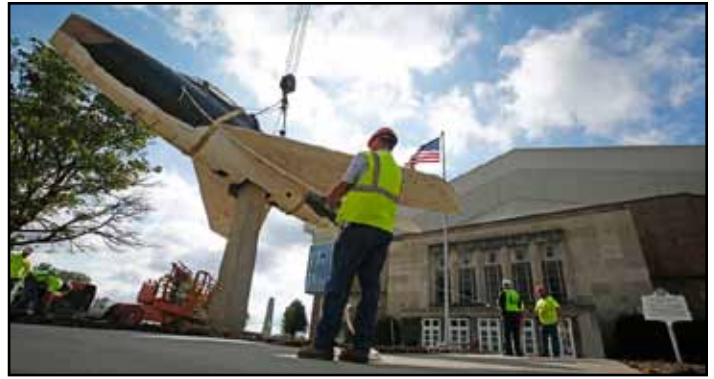
Crews from Weigand Construction and Martin Construction guide the F-84F Thunderstreak jet as it’s lowered onto its new pedestal in Memorial Coliseum’s new Veterans Plaza, which was dedicated Nov. 7.
