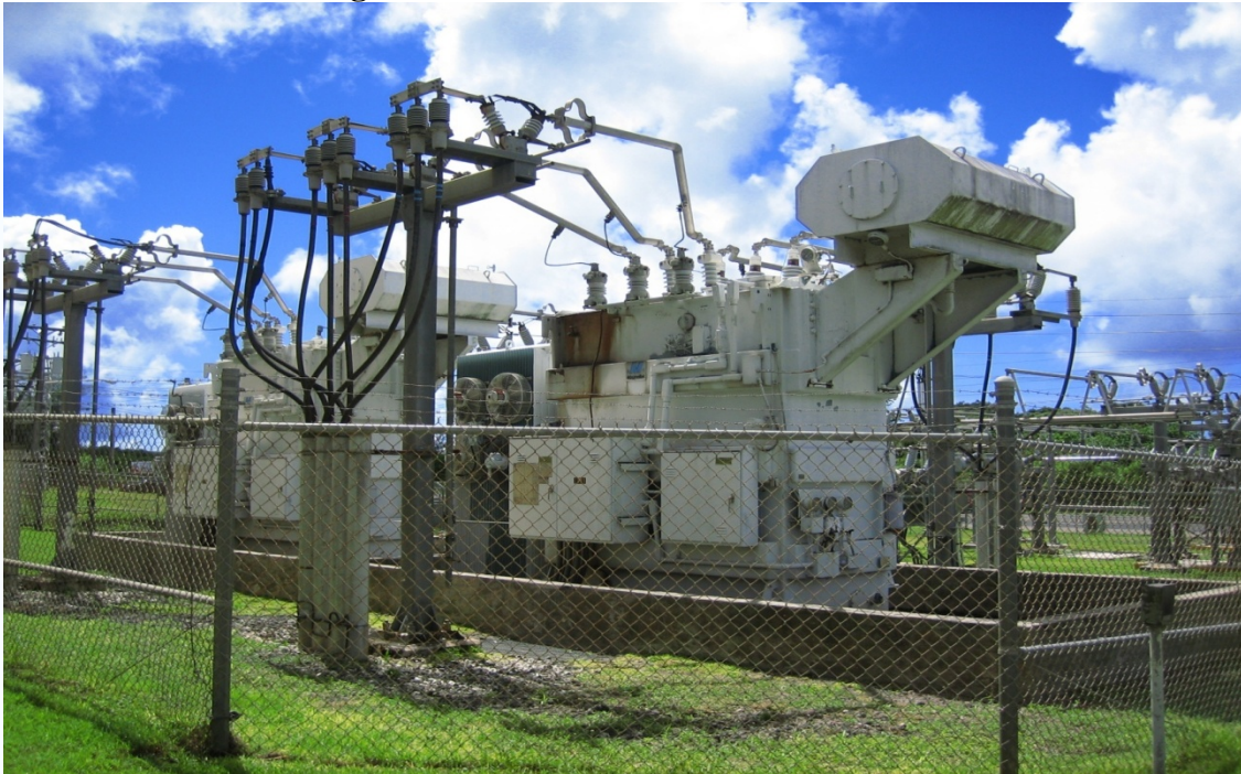
Figure 9. Harmon Annex Power Station
