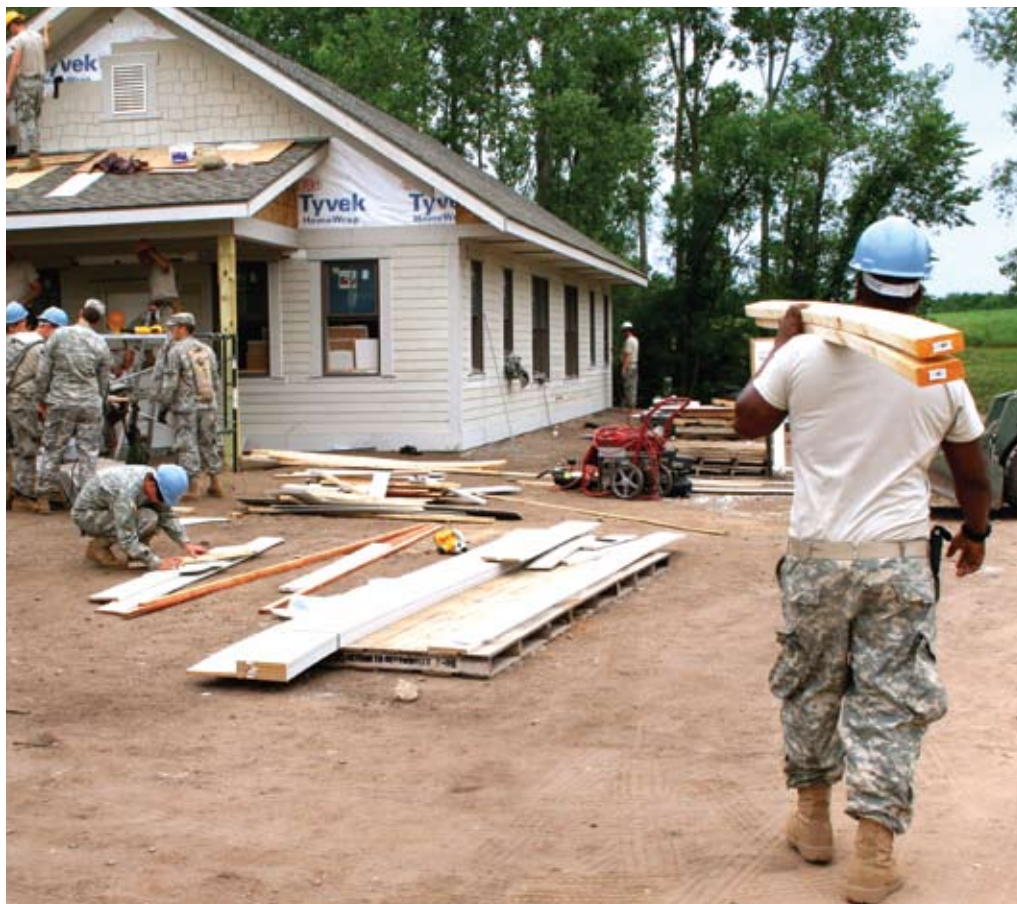
Left: PVT James of the 851st Vertical Engineer Company (right) delivers lumber during the construction of two Veterans' homes near Hugo, MN, June 24, 2009. The 851st Vertical Engineer Company is busy constructing new buildings and completing other various tasks during their two-week annual training.
