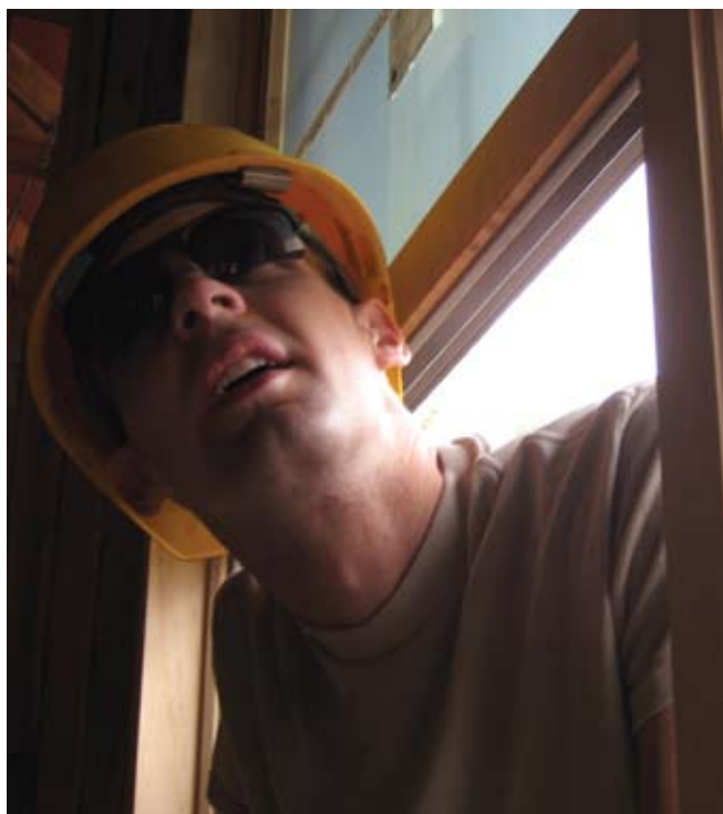
PFC Carl Swanson, a carpenter with the 851st Vertical Engineer Company, checks the interior of a new home for the Disabled Veterans Rest Camp in Washington County, MN, June 18, 2009.
