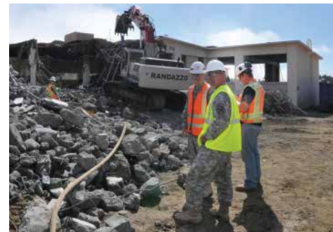
TOP: As recommended by the RCTMP, this Florida ARNG facility in Miami is slated for divestiture. BOTTOM: Demolition in progress.
