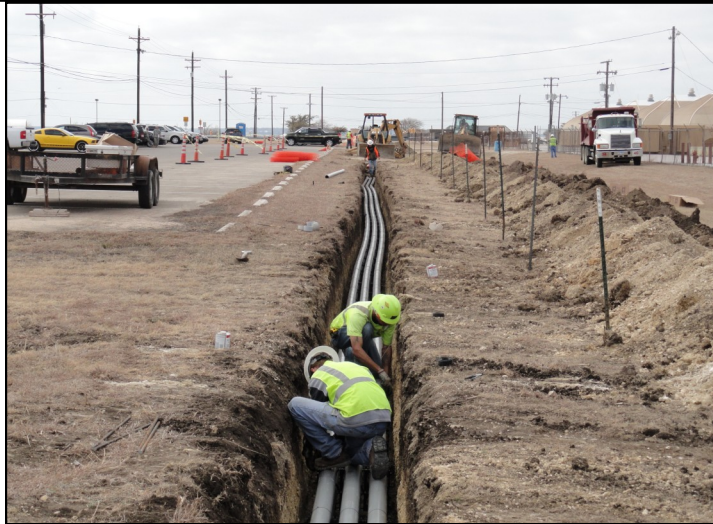
Contractors installing conduit as part of the $9.4 million infrastructure contract to support the construction of the new medical center. (Corps of Engineers Photo by Kevin
