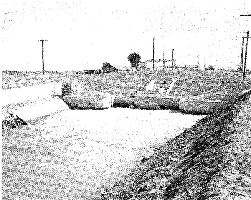
Figure 4-1. Tube Turbine Installation, Allis-Chalmers, 420 kW, 16.5 ft. head, 300 cfs, Turnip Power Plant (Courtesy Imperial Irrigation District, Imperial, California).
