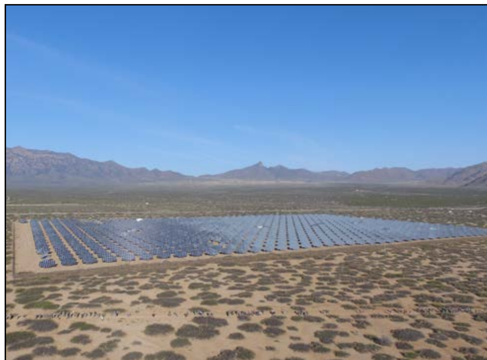
Solar pannels comprising WSMR's 42-acre solar array. (Photo: WSMR PAO)
