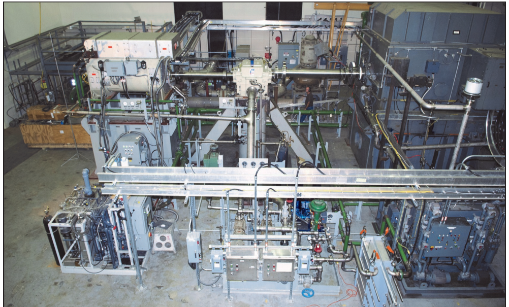
Naval Surface Warfare Center Carderock Division – Ship Systems Engineering Station (NSWCCD-SSES) engineers completed full scale testing of a 7,000-rpm, 14-megawatt High Speed Generator (HSG) at the Land Based Test Site (LBTS), Sept. 19. The prototype provides up to six times more power than lower speed, conventionally cooled, similar sized generators currently available. Photo by Martin Sheehan.
