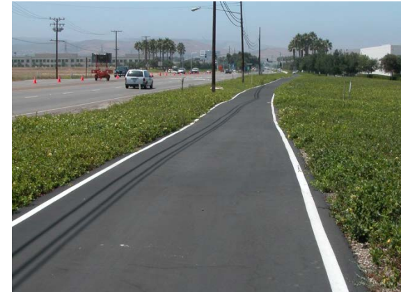
Detached paved sidewalk
