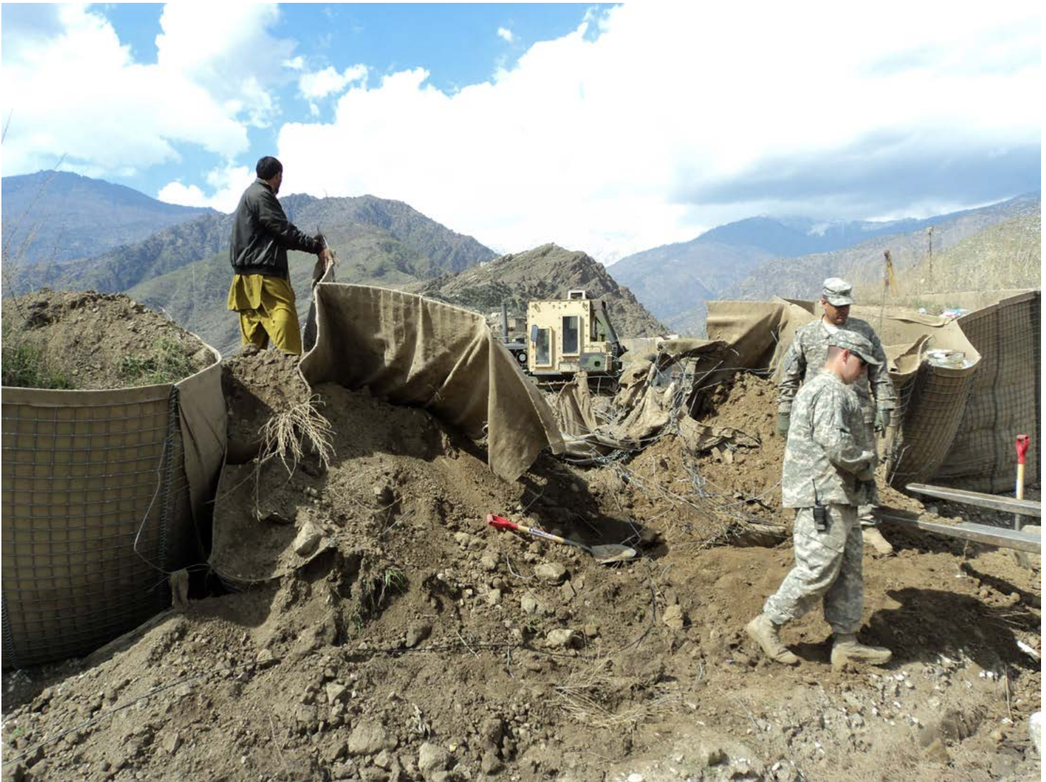
1LT Robbie Laufer and SFC Omar Soto work with local nationals in the construction of a new fire base on COP Honaker Miracle, Kunar province, Afghanistan. (Photo by 1LT Tommy Horne, U.S. Army)
