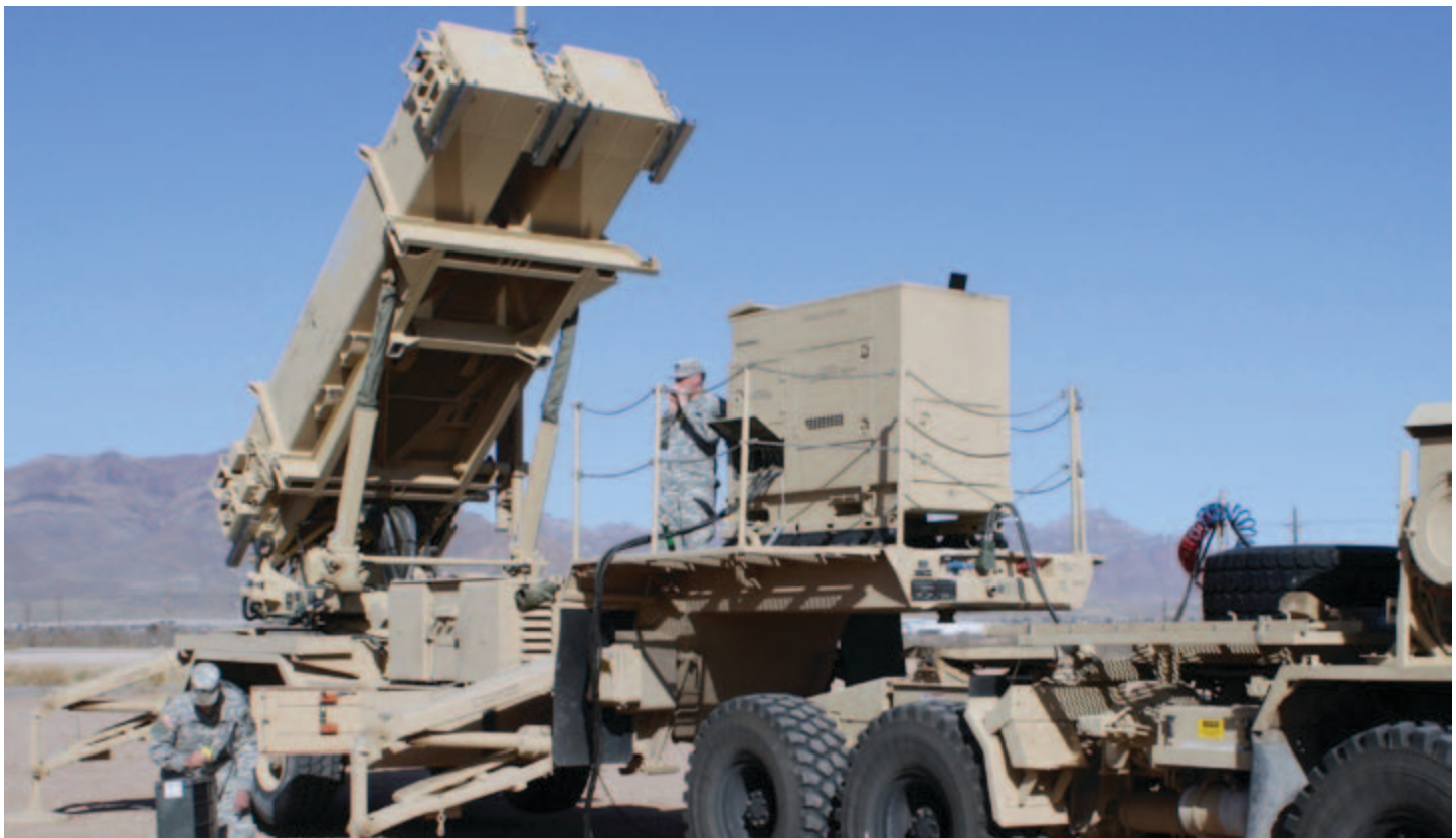
SPC Brian Deaton and PFC Edward Nedweski, power generation equipment repairers with 5th Battalion, 52nd Air Defense Artillery, perform a load bank test of a Patriot Launching Station generator during a week-long maintenance program. (Photo by CPT Dan Moore, U.S. Army)
