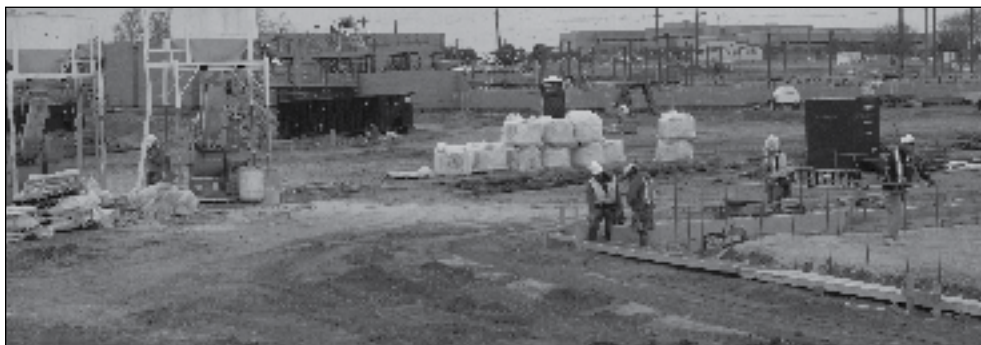
Construction workers on Fort Sill, Oklahoma, lay foundations at the future home of Air Defense Artillery. (Photo by Keith Pannell, the Cannoneer , Fort Sill)
