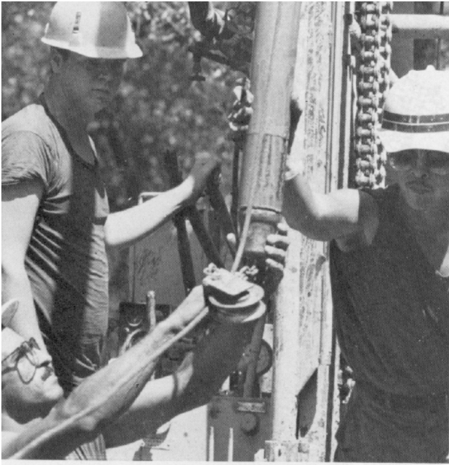
Members of a well-drilling crew remove a piece of the drilling section from the ground.
