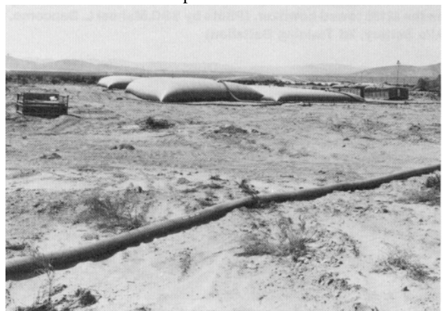
Six-inch hoseline and the 20,000-gallon fabric storage tank are part of the tactical water distribution set.
