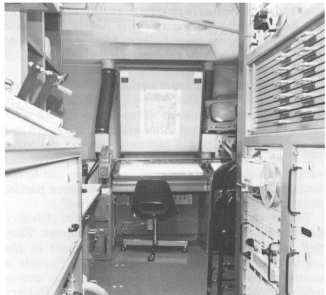
Interior view of the shelter showing the photo interpretation console and supporting computer and communication equipment.
