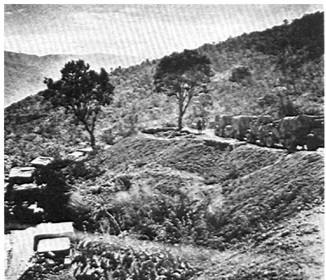
Figure 13. A road, complete with hairpin curves, was backed through the Chin Hills from Imphal to Tiddim.
