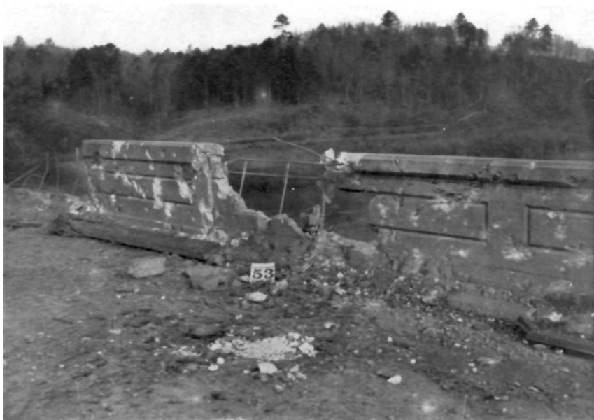
FIG. 3.—HIT OF 155-MM. SHELL NO. 20 IN ROADWAY (FOREGROUND). BOTH NORTH AND SOUTH PARAPETS WERE BROKEN
