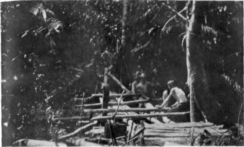
THE CONSTRUCTION OF NUMEROUS SHORT BRIDGES WAS BUT ONE ITEM IN THE TOIL OF THE JUNGLE TRAIL.
