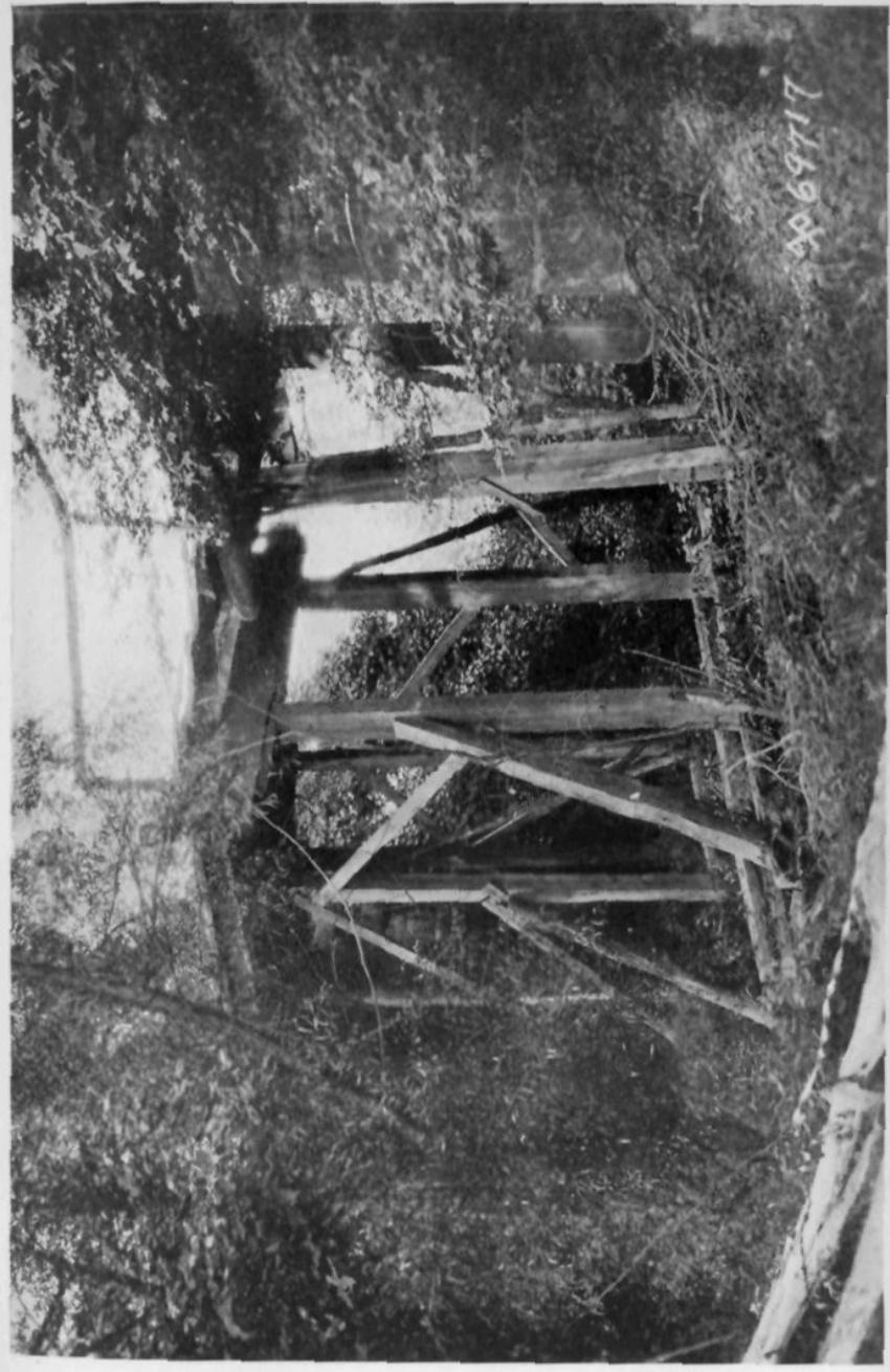
PHOTOGRAPH No. 4.—HIGH BRIDGE BROKEN BY 5-TON TRACTOR. (TIMBERS ROTTED OUT.)
