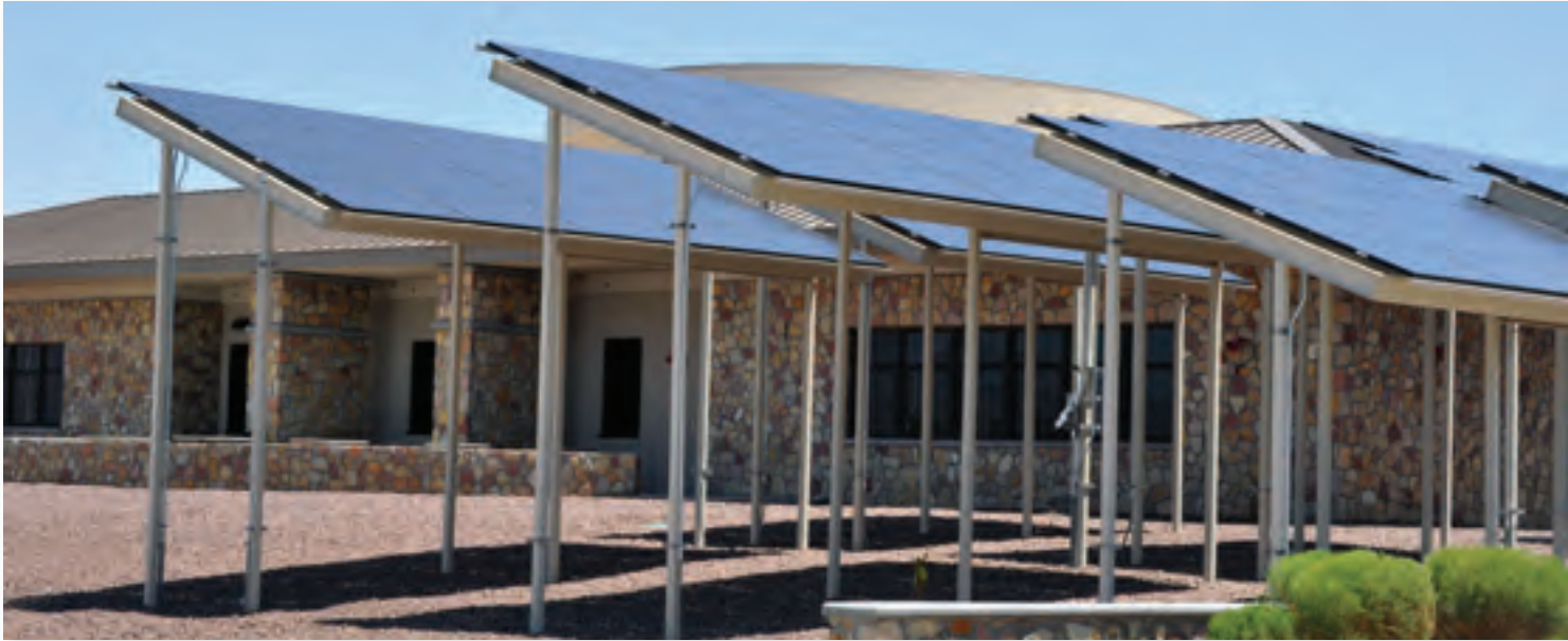
Solar panels at 4th Brigade Combat Team, 1st Armored Division Dining Facility on East Fort Bliss, Texas. (Photo by Samantha Reho)
