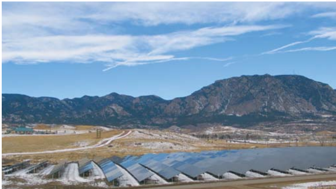
The Fort Carson Solar I array was completed in December 2007.
