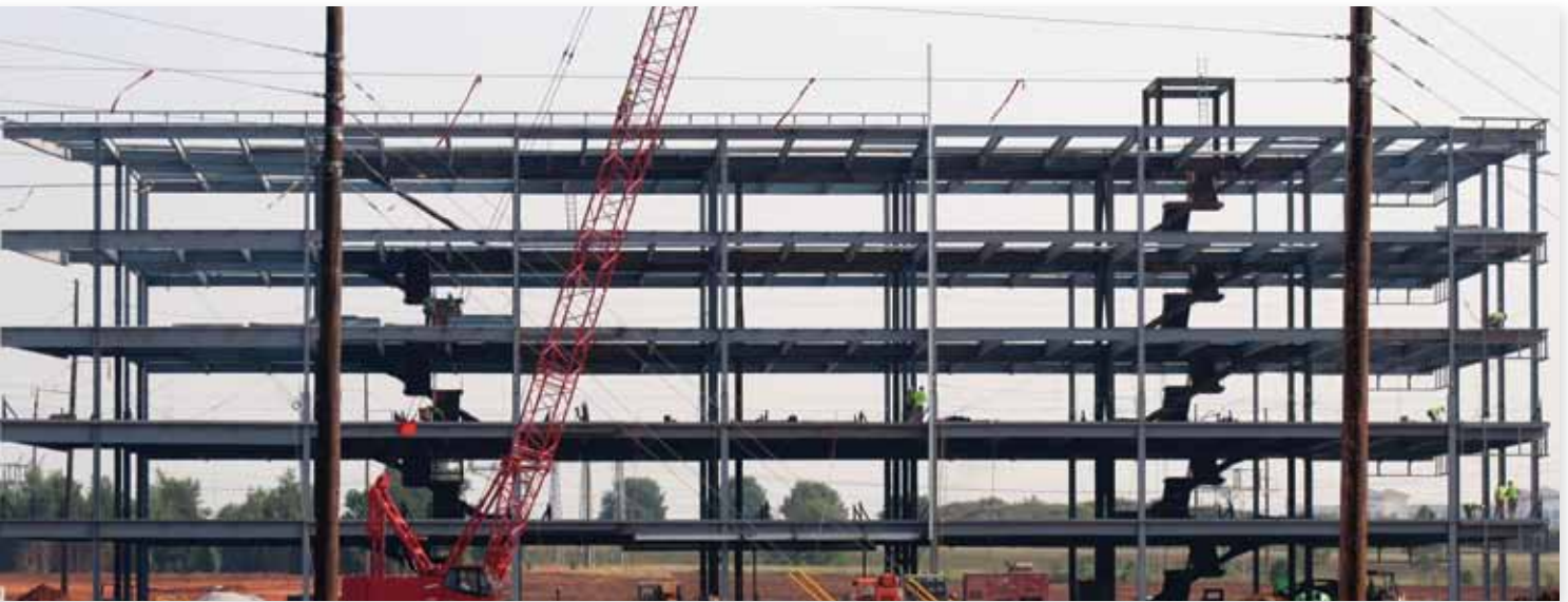
Ongoing construction for the initial building in the Redstone Gateway office park. This Enhanced Use Lease project is the result of the partnerships between Redstone Arsenal, the city of Huntsville, Madison County and state officials as well as the development team of COPT and Jim Wilson & Associates.
