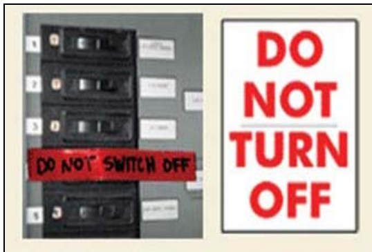
Label circuit breakers in fuse box
