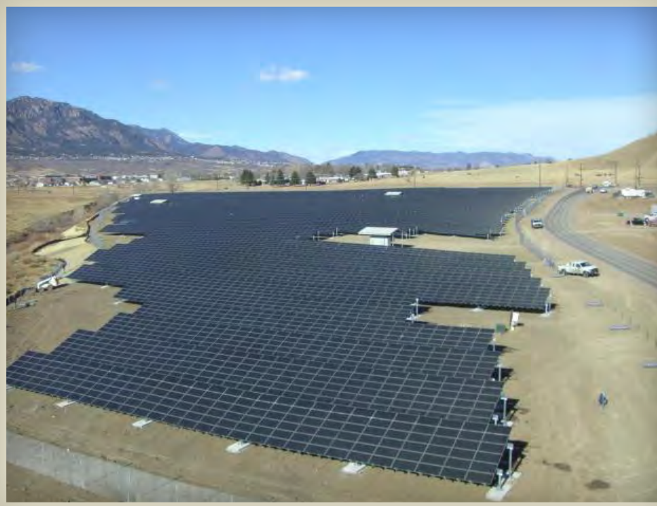
Photovoltaic solar array - Fort Carson, Colo.
