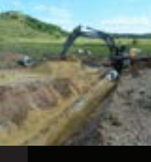
JMRC HOHENFELS Mitigate Safety Obstacles; Erosion Control Areas A, B, and C; Tactical Valley Crossing Repair; Maneuver Corridor Repair
