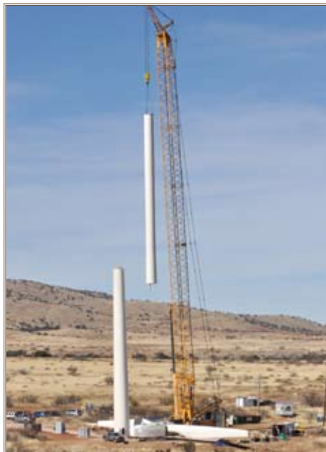
The crane crew hoists the top half of the 70-meter wind turbine tower into place on Fort Huachuca. Photos by Daniel J. Calderón
