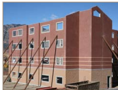
At the Warrior-in-Transition barracks, a four-story precast wall panel is placed, completing the building's exterior early in construction.
