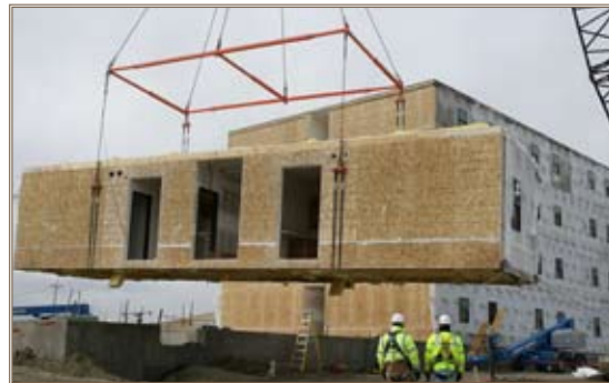
Modular units containing two suites with fixtures, cabinetry and doors are hoisted into place at the brigade combat team-heavy barracks. Photos by Harry Weddington
