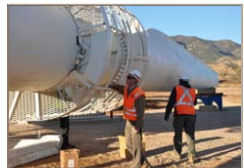
Mike Brown (left), project engineer for the Corps' Fort Huachuca Office, and an unidentified man take a look at the nacelle for the wind turbine before it is lifted into place.
