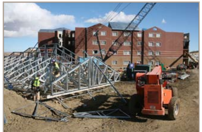
Workers prepare preassembled roof trusses for lifting by cranes onto the WTB roof at Fort Carson. Photo by Chip Kossow
