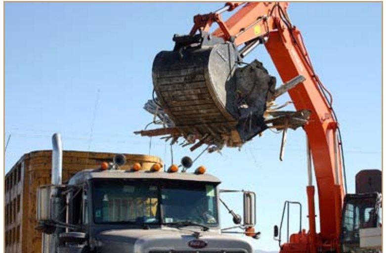
An excavator looks like a Tyrannasaurus Rex as it “eats” the building and drops the debris into a dump truck for removal to the landfill. Photo by Debra Valine
