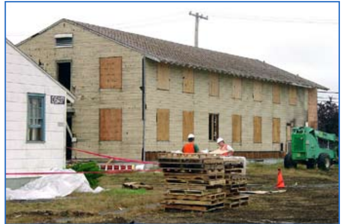
During the deconstruction process, World War II buildings at Fort Lewis, Wash., are stripped of their first layer of siding. The white building at left is an example of a World War II building that is representative of their current state.
