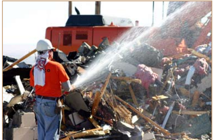
Jose Avalos, ICONCO/LVI Demolition Services, keeps the building wet during demolition to ensure particles of asbestos are not released into the air. Photo by Debra Valine
