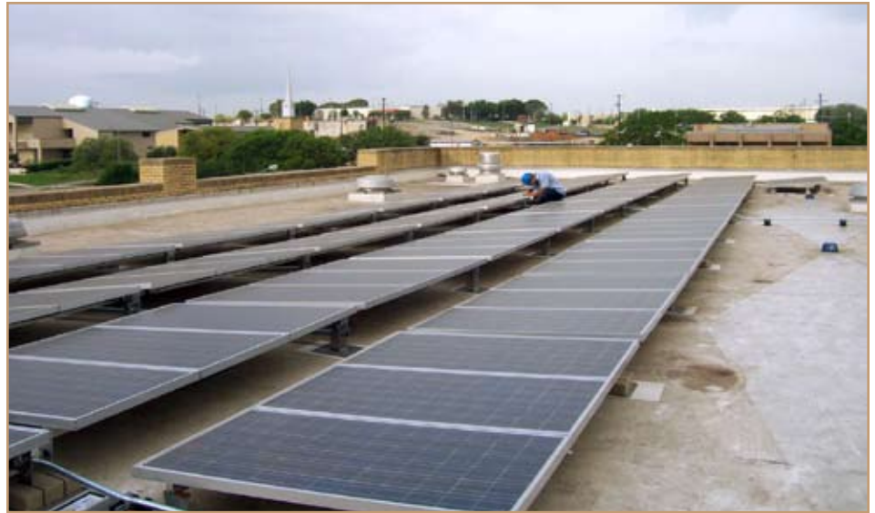
A worker installs photovoltaic solar panels on Bldg. 1350 at Fort Sam Houston, Texas. The panels augment electricity from the local power company and are saving the installation nearly $6,000 a month in energy costs.
