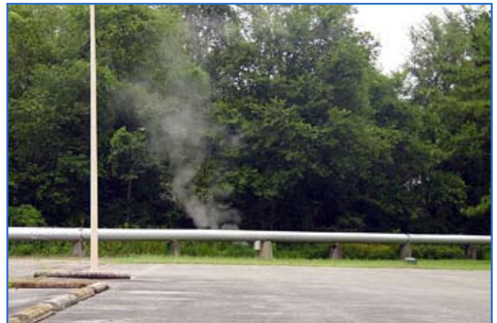
A system leaks steam at Redstone Arsenal, Ala. The system was part of a central energy plant assessment. Photo courtesy of Pacific Northwest National Laboratory
