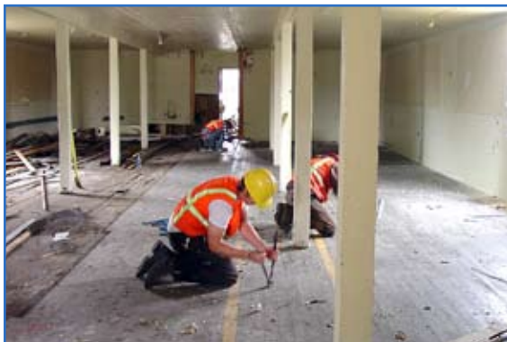
Contractors remove reusable products for resale in the marketplace. Resale of recovered materials allows the contractors to recover much of the labor costs associated with deconstruction.
