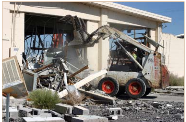
Alex Villalazo, ICONCO/LVI Demolition Services, picks up the smaller pieces of debris with a bobcat. Photo by Debra Valine
