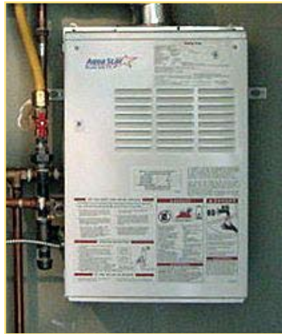
Tankless water heaters like this one have been installed in family housing units at Fort Lee, Va. Photo by Jerry Martin.
