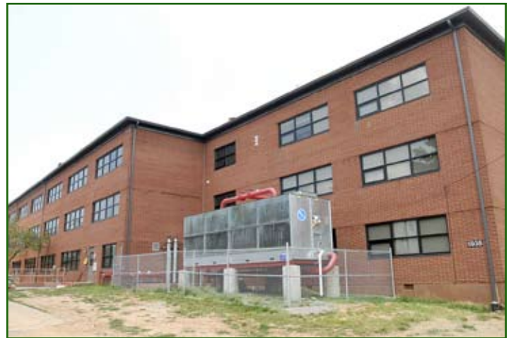
An earth-coupled/hybrid cooling unit provides peak cooling for the buried parade field loop. Photo by Stephen Moore
