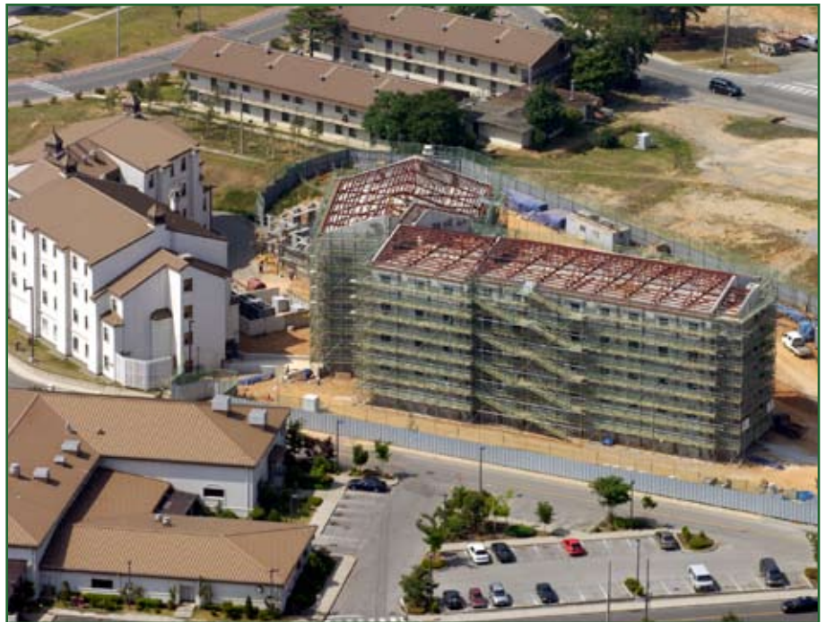
The new extension to the Humphreys Lodge will double the number of rooms in the facility and include conference space and other amenities to support a variety of training, temporary duty and recreational needs. Photos by Edward Johnson
