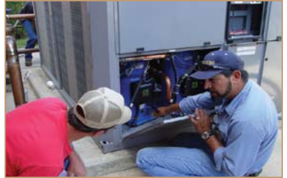
Gary Shuffler and Tommy Figueroa (left to right), DPW Maintenance Division, make adjustments to controls of the newly installed chiller. Photo by Virginia Sanders.
