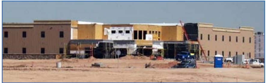
Brigade Combat Team facilities construction is underway at Fort Bliss, Texas. Photo by Dennis Ballog
