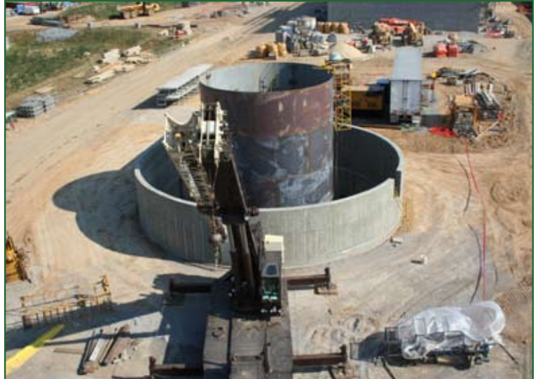
The Commercial Cogeneration Power Plant EUL project at Fort Detrick, Md., involves about 10 acres of the National Interagency Biodefense Campus on the main post. The developer, the Chevron-Texaco/Keenan Development Team of Washington, will operate and maintain the plant and provide an in-kind consideration to the Army equal to the fair market value of the leased assets. Photos courtesy of U.S. Army Corps of Engineers, Baltimore District
