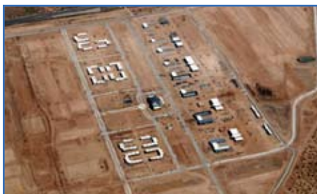
This aerial photo taken in October shows Brigade Combat Team facilities under construction at Fort Bliss, Texas. Photo courtesy of the Fort Bliss Master Expansion Program Team
