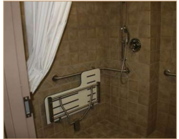
Before renovations, the bath held a regular bathtub. With the changes, wheelchairs can easily roll into the shower allowing a measure of safety and normalcy for wounded warriors. Photo courtesy of Fort Sam Houston, Texas, Public Information Office
