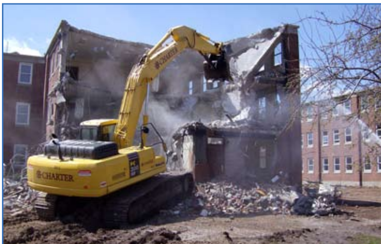
Charter Environmental begins the second phase of demolition of Building 408 at Fort Hamilton, N.Y. Huntsville Center's Facilities Reduction Program is working with the installation, New York District and contractor partners to remove three buildings. Photo by Kevin J. Merenda, New York District, U.S. Army Corps of Engineers
