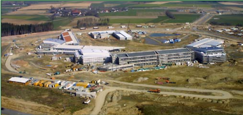
An aerial overlook flight of Germany's Grafenwöhr installation in March 2007 reveals Netzaberg Village's MILCON Island projects, including elementary and middle schools, a child care center, a youth activity center, a chapel, ball fields and a new infrastructure network. The U.S. Army Corps of Engineers, Europe District, is managing the construction of this project.
