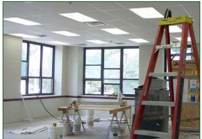
At Picatinny Arsenal, N.J., facility space located inside its mission critical area is being redeveloped for lease under an EUL. Six warehouse-sized buildings on the roughly six-acre site have been demolished. Three new structures totaling 125,000 square feet will replace the old. The developer, InSitech, will also develop and lease a 1.1 million square-foot facility, the Picatinny Applied Research Campus, on 120 acres of land.
