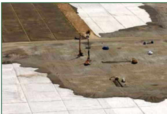
Construction has already started on newly acquired land adjacent to Camp Humphreys. Before engineers can build on the former rice paddies they must first drain them of water; conserve the topsoil, seal the surface with a porous barrier and raise the ground with fill material.
