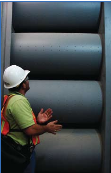
Mitch Duke, technical engineer for the Pentagon renovation, inspects the new filters for the Pentagon's heating, ventilation and air conditioning controls system. Photo by Andrea Takash
