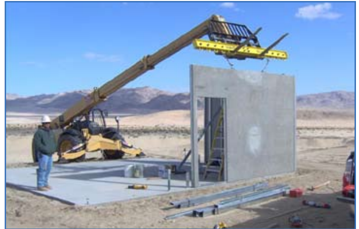
Employees with RQ Construction Company, Bonsall, Calif., build the Jabal Military Operations Urban Terrain training site at Fort Irwin, Calif., using studcast panels versus traditional steel and concrete construction. Photo by Capt. Seth Henson
