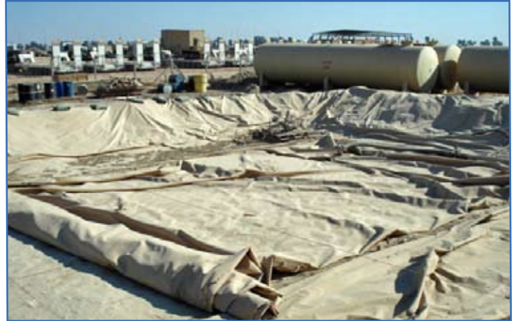
A fuel soaked bladder sits in front of more mobile skid-mounted fuel storage systems. Photo courtesy of 249th Engineer Battalion (Prime Power)
