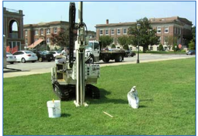
Contractors conduct field sampling activities at Fort Monroe, Va. This sampling is one of the many forms of sampling conducted across the nation as part of the ECP program. Photo courtesy of U.S. Army Corps of Engineer, Louisville District
