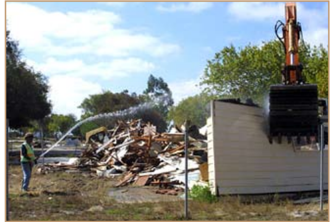
A construction worker hoses down a section of a house to keep dust from flying as it is torn down. Photos courtesy of U.S. Army Corps of Engineers, Los Angeles District
