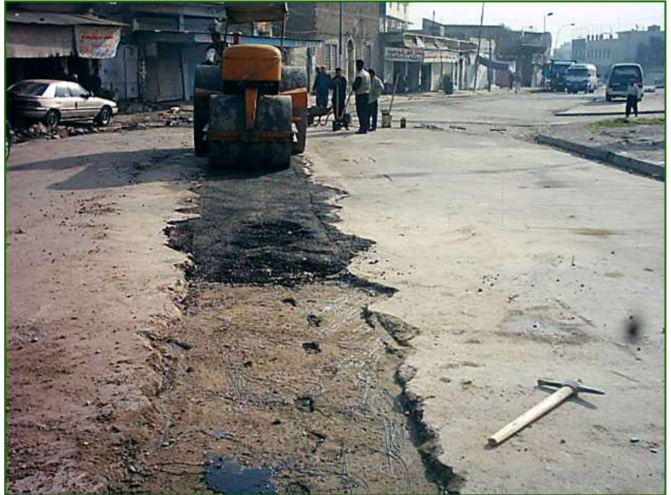
Road surface is replaced following the installation of new sewer pipes in Mosul. USACE file photo
