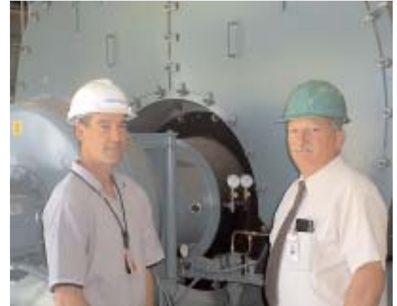
Richard Havrisko (Right) and William F. Porphy, Facilities Operation Manager, Chevron Energy Solutions, inspect a Cleaver-Brooks 500-hp boiler.
