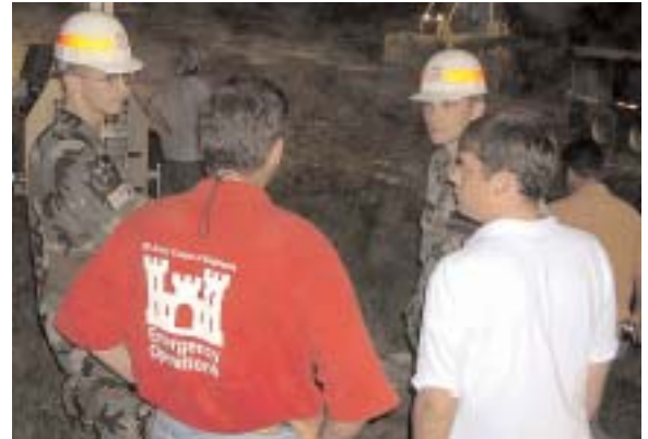
With Hurricane Rita approaching the Gulf area, construction crews work around the clock to reinforce an interim levee repair that was made after a breach caused by Hurricane Katrina. A USACE Quality Assurance team from Task Force Unwatering was on site at the St. Bernard Parish back levee location. Left to right; Capt. Jason Wood, Kevin Wagner, Capt. David Pounds and Benjamin Farrell. (Photo by Hank Heusinkveld, Wilmington District, USACE)
