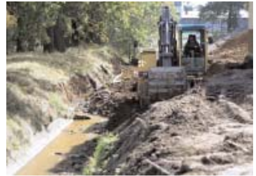
A backhoe is used to remove dirt and concrete and to widen the banks of a small stream running through the 284th Base Support Battalion in Giessen, Germany.
