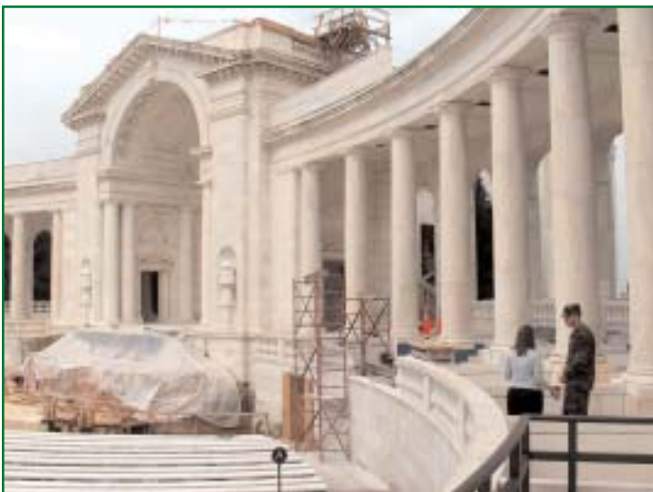
The U.S. Army Corps of Engineers began work in March 2005 to refurbish and repair the amphitheater reception building. (Photo by Chris Augsburger)
