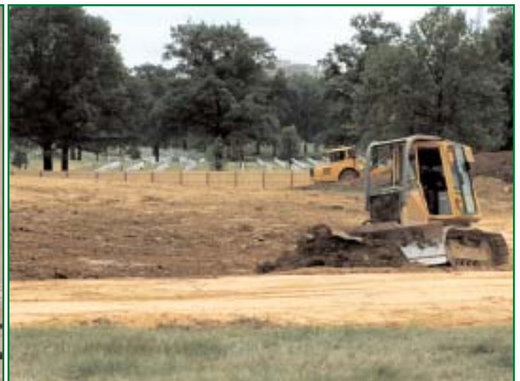
A contractor grades 40 acres of open land for new interments. The project, which is called Land Development 90, will open in 2007 and provide 20,000 to 30,000 new gravesites. (Photo by Chris Augsburger)
