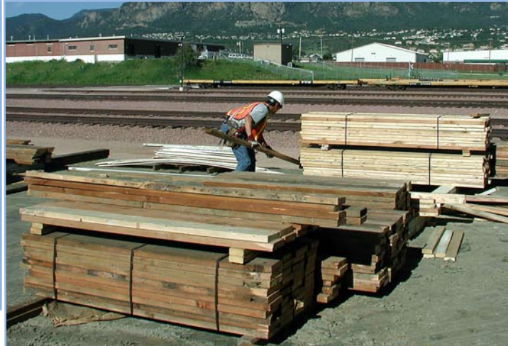
Lumber from a deconstructed warehouse is bundled and banded to be sold at a used building material retail business.
