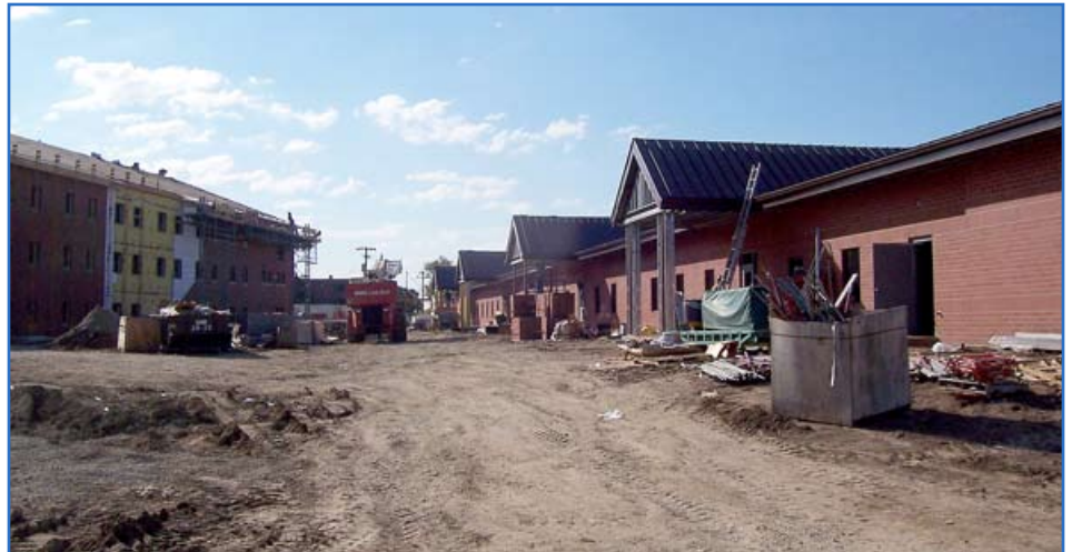
Barracks being constructed at Fort Riley, Kan., will support the 10,000 Soldiers expected to arrive by the year 2011. The increase of Soldiers is a result of the BRAC closing military installations in Germany and moving the 1st Infantry Division headquarters to Fort Riley. (Photo courtesy John Schreiner)
