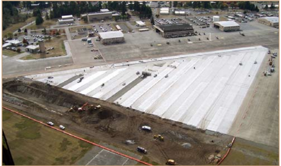
As part of the Modularity Program at Fort Lewis, Seattle District constructed a helicopter parking apron at Gray Army Airfield. The large excavation is for a stormwater detention vault. (Photos by Thomas Poole)
