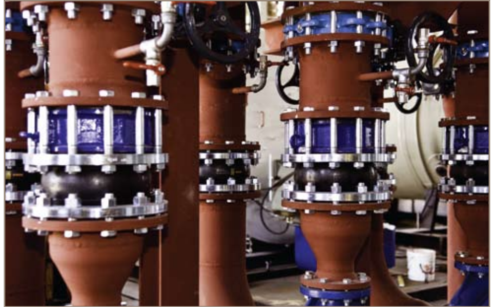
Newly installed pumps at Camp Ederle in Vicenza, Italy, are the first completed portions of the Energy Savings Performance Contract to install new boilers and a cogeneration unit on the installation. Photo by John Rice, U.S. Army Corps of Engineers.
