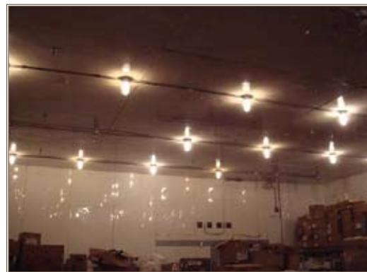
Incandescent light fixtures in a Fort Meade commissary freezer room consume considerable amounts of energy. Photo by Energy Focus Inc.
