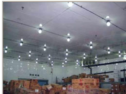
LED lights installed in the freezer room for a demonstration project consume less energy, provide more light and will have to be replaced less frequently. Photo by Steven Parker
