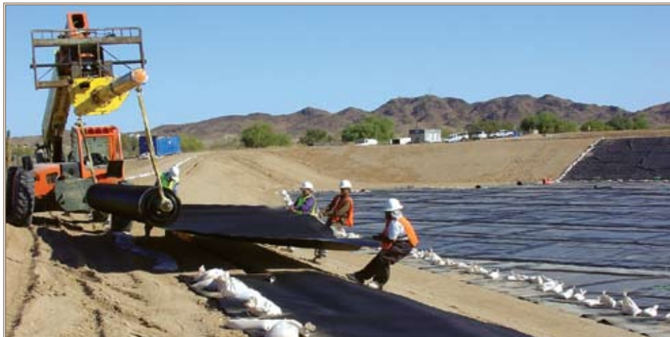
Construction crews roll out hundreds of feet of high-density polyethylene geomembrane lining at the sewage lagoons. Photos by Mary F. Flores
