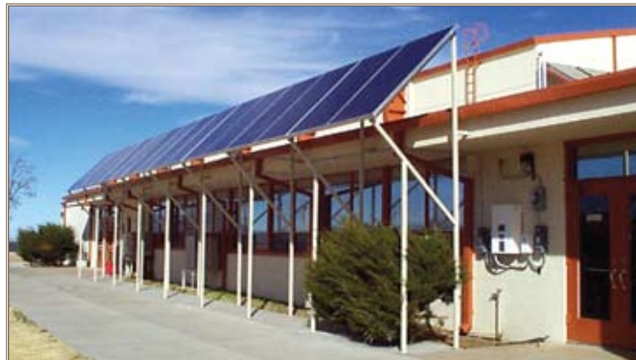
Photovoltaic panels at work at Fort Huachuca, Ariz. Photo courtesy of Bill Stein
