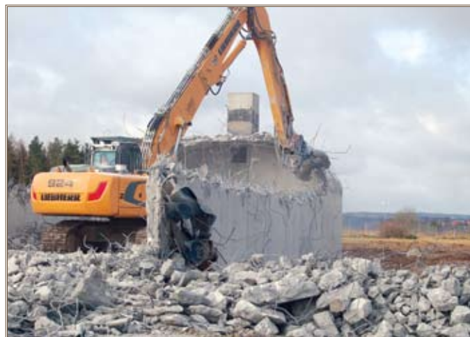
German contractor BG Werning/Weibrauch use heavy equipment to demolish concrete portions of an old bunker at Urlas, Germany. Photo by Norman Cotter
