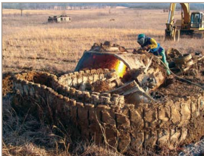
EOD Technology's scrapping subcontractor, Tyne Earth and Demo, finishes cutting apart the turret of an M-60 tank. Photo by William Noel
