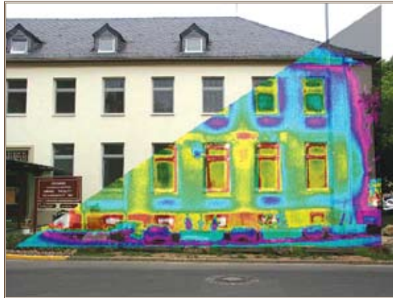
USAG Schweinfurt's Energy Savings Program included thermographic analysis of buildings. Composite of photo by Kai Battenberg (AMEC Earth&Environmental) and thermographic image by CPWeber GmbH
