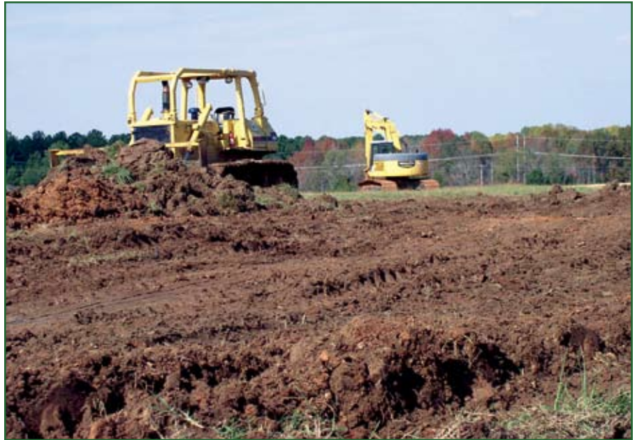
Remediation efforts to correct leachate pops are underway at Woodlawn Landfill on Fort Campbell. Photo by Richard Huser, Fort Campbell Solid Waste/Recycle Program contractor
