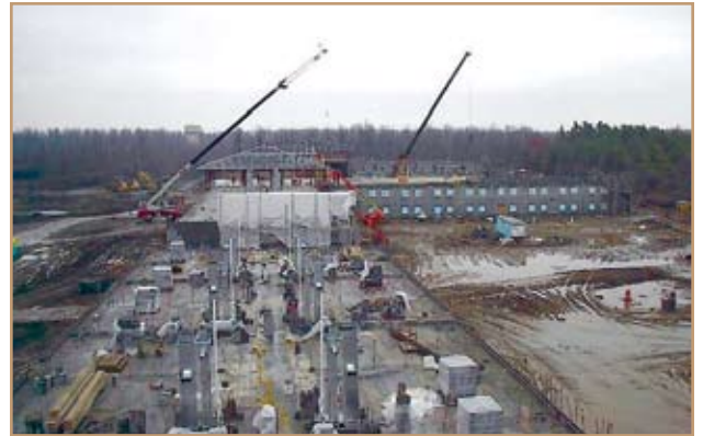
New barracks are under construction at Fort Drum. Photo by Mark McKenna, U.S. Army Corps of Engineers New York District
