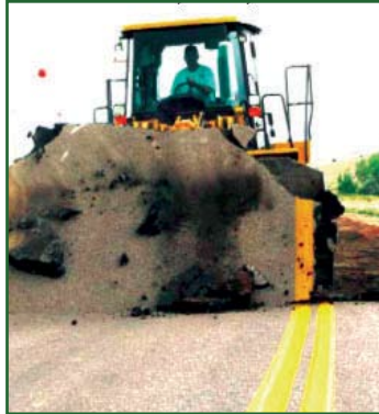
A worker removes the pavement from Brown Road at Fort Carson, Colo., as part of the initial construction project to prepare for the arrival of the 4th Infantry Division. Photo by Sgt. Clint Stein
