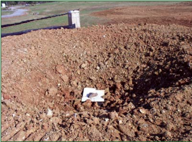
A folder marks the spot where an extraction well that will remove leachate is to be constructed at Fort Campbell. Photo by Richard Huser, Fort Campbell Solid Waste/Recycle Program contractor
