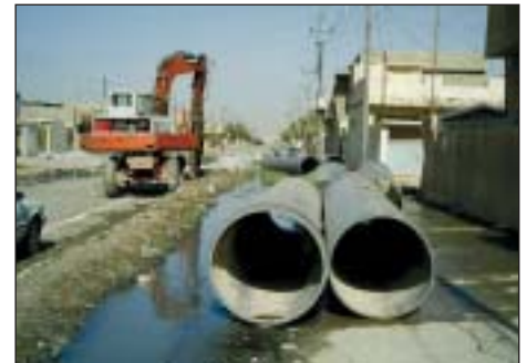
Pre-positioned pipe and marked trench lines together with the trencher in position, are positive signs for local residents that a new sewer system will replace the open sewer also shown.
