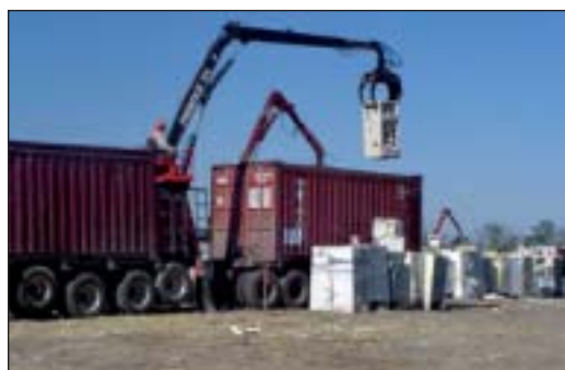
Debris that may contain hazardous substances, such as refrigerants, are separated from the rest of the waste. (Photo by Mary Beth Hudson, USACE)
