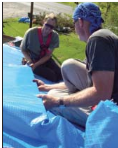
The Corps has installed more than 60,000 temporary patches under FEMA's Blue Roof program. (Photo by Matt Craig, Memphis Commercial Appeal. Used with permission.)
