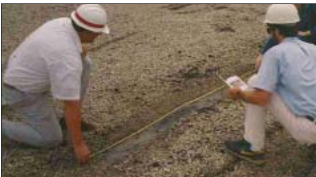
Roof inspections can be combined with infrared survey data to manage roof M&R.
