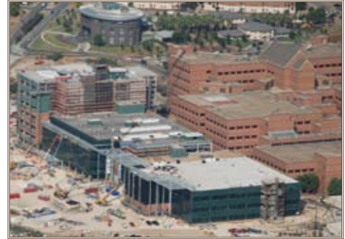
New SAMMC facilities are under construction at Fort Sam Houston. Photo courtesy of U.S. Army Health Facilities Office
