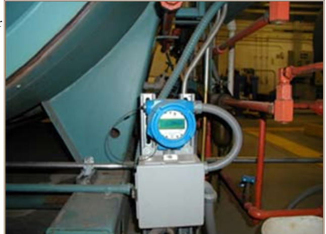
An oil meter measures fuel usage for boilers at Fort Hood. Photo courtesy of ERDC
