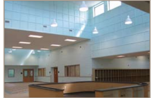
The main atrium of the School Age Center at Schofield Barracks features skylights that take advantage of Hawaii's abundant sunlight. Photos by Vanessa Lynch
