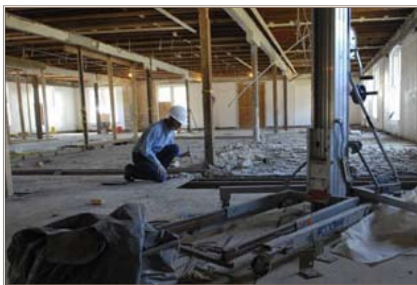
Chantal McKenzie determines if crawlspace clearance meets applicable building codes in a historic building undergoing major rehabilitation at Camp Mabry, Texas.
