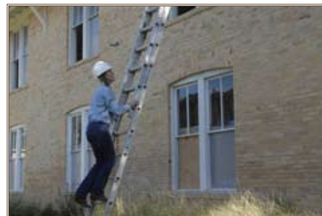
Chantal McKenzie assesses exterior mortar removal techniques performed by a masonry subcontractor to ensure protection of historic bricks. "Photos courtesy of Texas National Guard"
