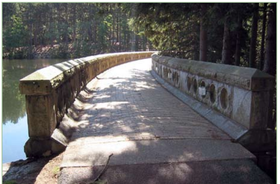
The walkway at Lusk Reservoir Dam. Photo by Milton N. Ricks, Project Engineer, U.S. Army Corps of Engineers, New York District
