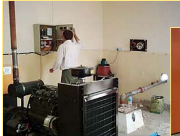
The operations technician checks gauges in the Al Maman pump house. In the foreground is the generator engine and pump, center is the well-head and water pipe running through the wall to the water tank, in the corner is the chlorinator.
