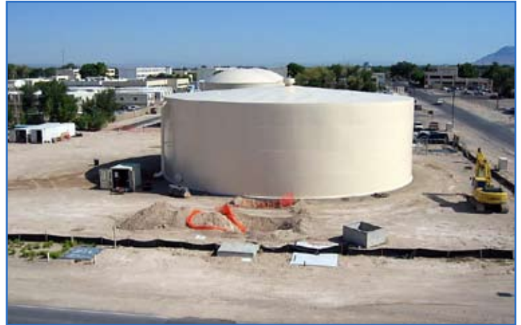
The Corps and Kirtland AFB worked together to produce the water treatment facility on base that now reduces arsenic levels to new EPA standards. Photos by Bruce Hill, Jr.
