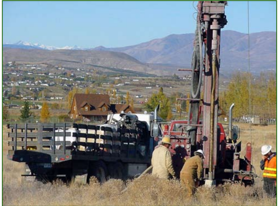
Groundwater monitoring wells are installed as part of an in-house site investigation at a Yakima Training Center environmental restoration program site.
