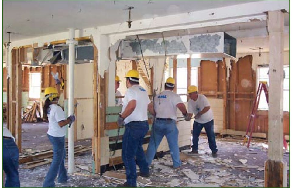
A crew of Habitat for Humanity volunteers salvages usable building materials from an excess Army barracks building at Fort Hood, Texas. Photo by Jeff Salmon, Fort Hood Department of Public Works, Environmental Division
