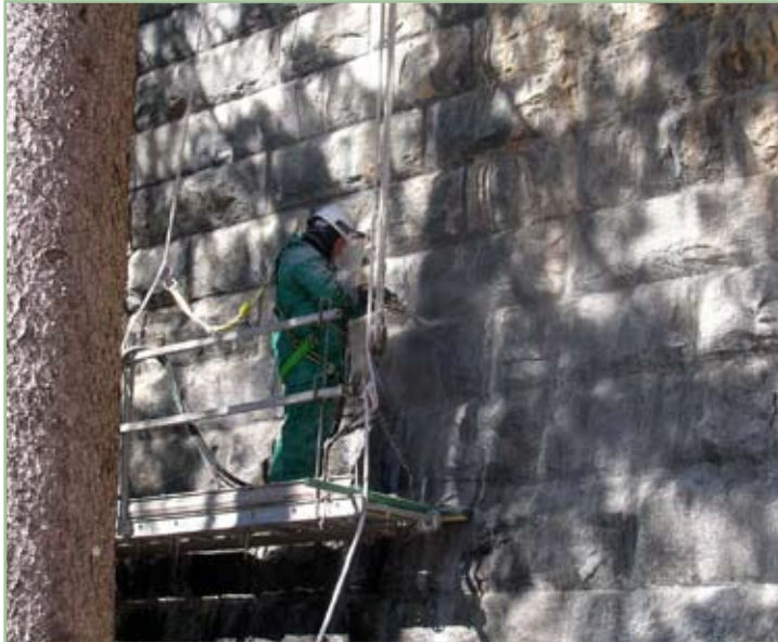
A worker cleans the calcite build-up on the dam's masonry stones by sandblasting them with small coarse grained silica, glass-like particles, under water pressure. Photo by Milton N. Ricks, project engineer, U.S. Army Corps of Engineers, New York District
