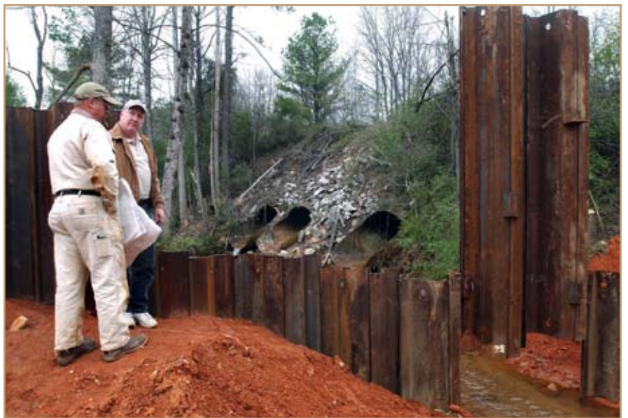
Ray P. Lambert Jr., of the Lambert Company, and Alan Miller, a project manager with the Corps’ Savannah District, view wetland mitigation efforts in Clayton County, Ga. Photo by Jonas Jordan, photographer, Savannah District
