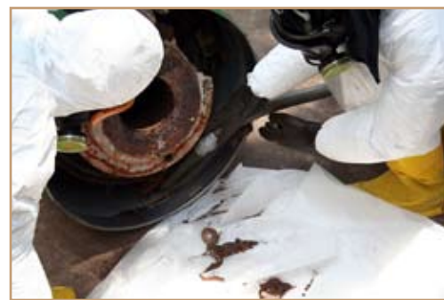
Contractors using a special vacuum collect liquid mercury that leaked out of a distribution head while being placed in a hazardous materials container. Photo by Patrick Bloodgood
