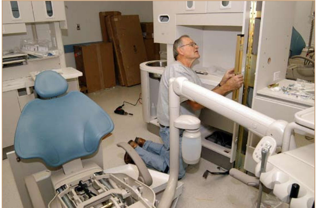
Ron Gaumer, a contractor with Austin Dental Equipment Company, ensures newly installed cabinets are in alignment during the final phase of renovation at the Camp Walker Dental Clinic. Photo by Galen Putnam
