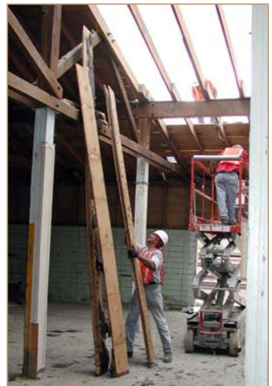
Materials are salvaged for reuse during the deconstruction of a World War II era warehouse at Fort Carson, Colo. Photo by Tom Napier
