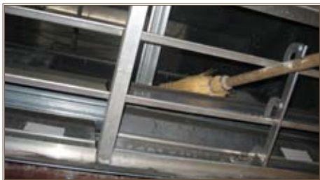
Occurrences like this in which a broom is used to physically override the control system can cause significant energy loss. Photo by Carl Lundstrom, EMC Engineers Inc.
