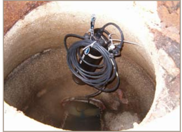
A flowmeter and data recorder installed in a manhole record wastewater study data. Photos courtesy of Pipeline Analysis LLC
