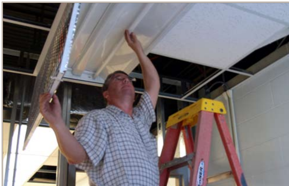
Lights are replaced with energy-efficient lighting, an example of a possible EEAP recommendation that can be phased in over five years and tied into the installation's energy reduction goals. Photo courtesy of ERDC-CERL
