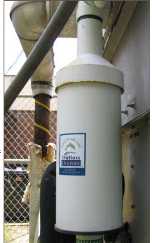
Fort Benning is using a chemical-free water treatment device at the Sand Hill PX. Photo by David Jenkins
