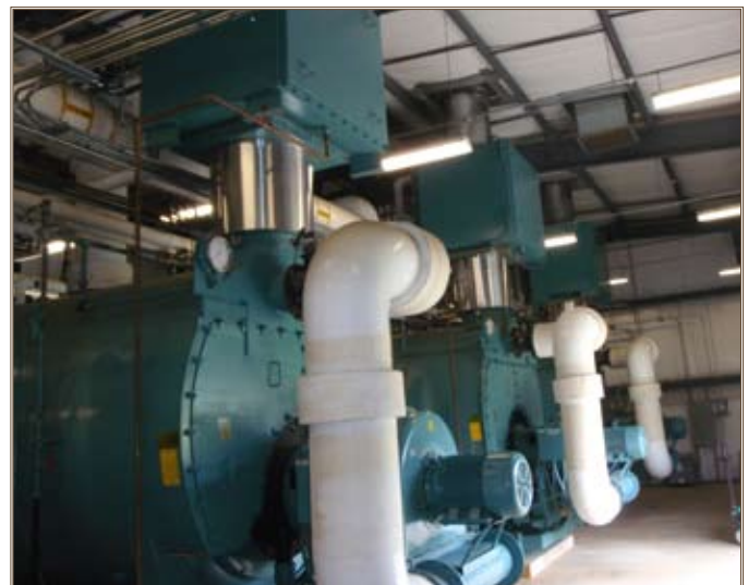
The recovery devices, the cubic blue boxes on top of each boiler stack, preheat water before sending it into the boiler as feedwater. Photo by Nick Stecky
