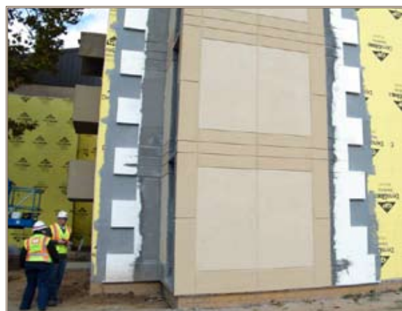
Engineers check the installation of the exterior insulation finish system. Photo by G. Valla
