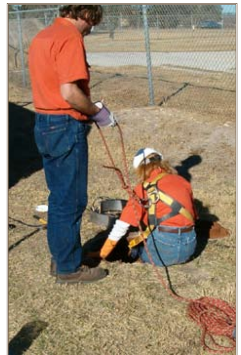
A technician descends into a manhole for the manhole and mainline assessments
