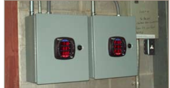
Advanced meters tracks electricity usage at Redstone Arsenal, Ala. Photo by Patrick Holmes, Johnson Controls, Huntsville
