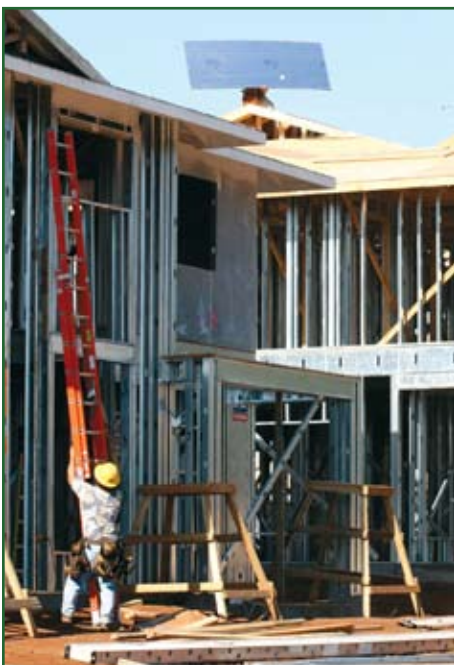
Workers add sheets of plywood to the roof on a duplex unit.
