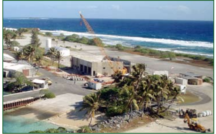
A crane aids construction of the Vehicle Paint and Prep Shop on Kwajalein Atoll in the Pacific Ocean. Photo courtesy of U.S. Army Corps of Engineers, Honolulu District
