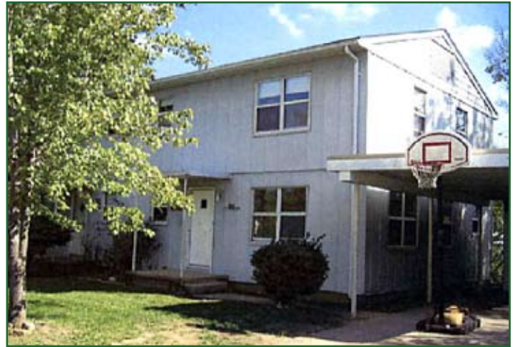
This three-bedroom duplex was selected for deconstruction at the Fort Leonard Wood privatized housing development. Photos courtesy of the National Defense Center for Environmental Excellence
